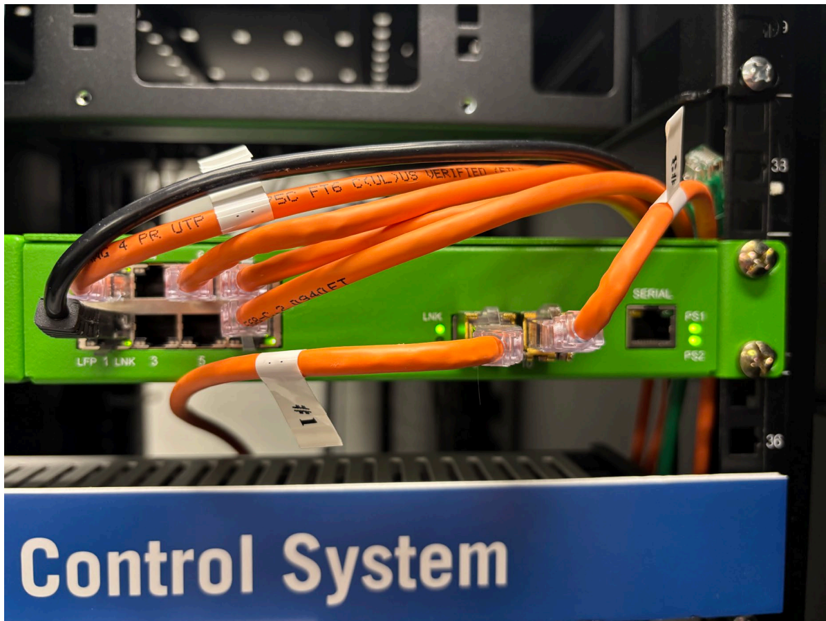
1909 Figure 4-72: Garland hardware configuration
